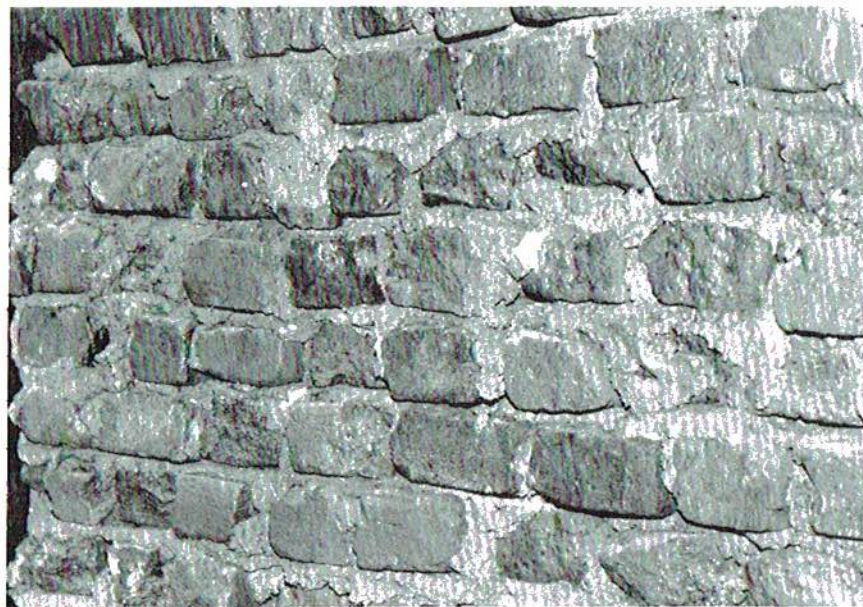
A portion of the original slave-made bricks have been exposed on the screened porch of the Beeson-Crow home.
